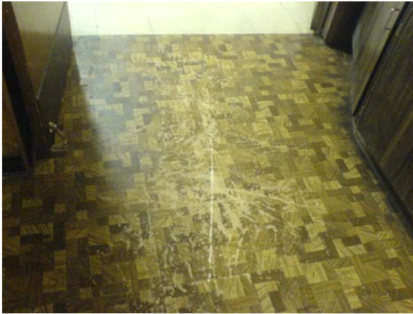
Old damaged floor
