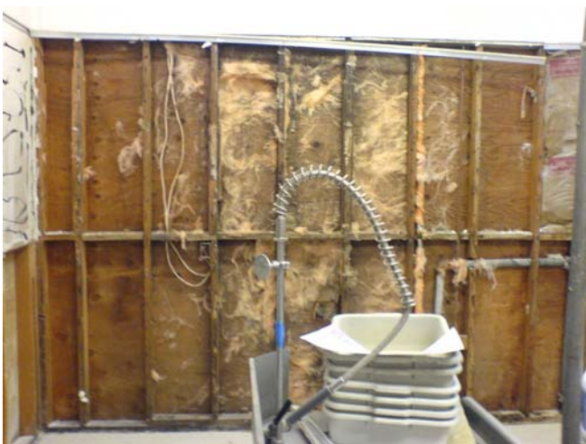
Old water damaged kitchen wall
